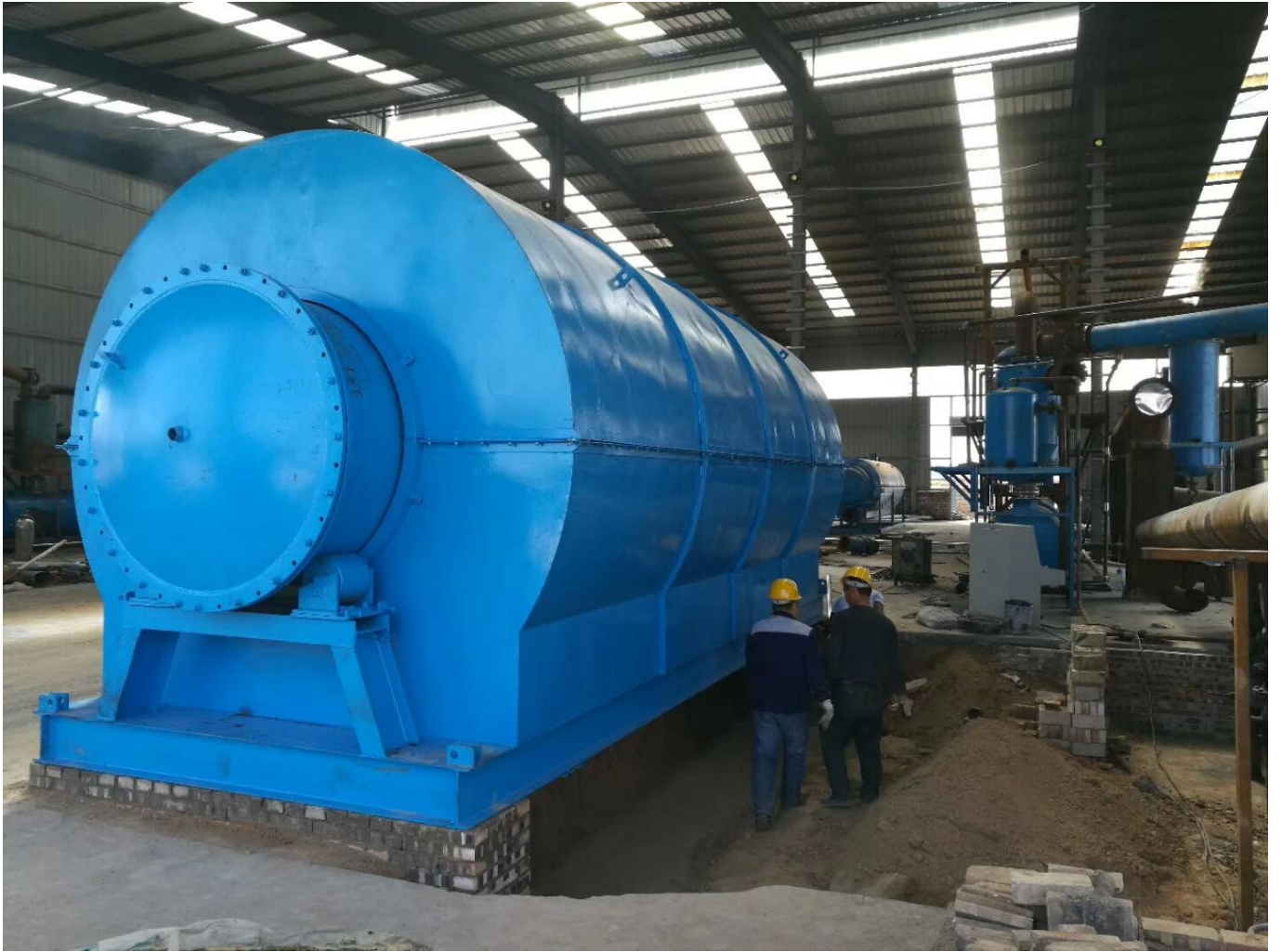
Batch type pyrolise equipment
