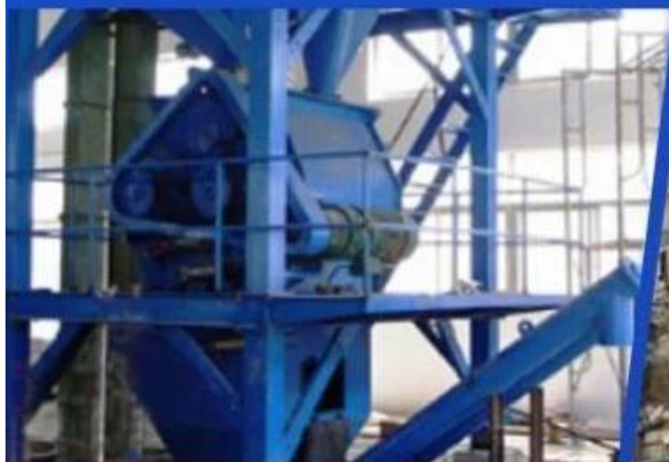
Waste incineration plant
